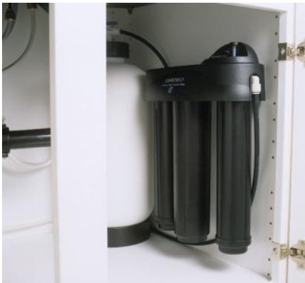
A KINETICO RO system showing membrane module & separate pure water storage tank in under sink kitchen cupboard.
