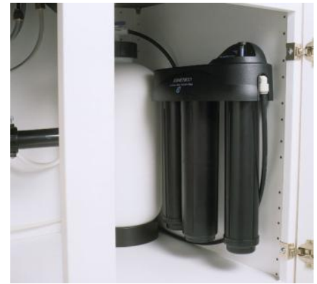
A KINETICO RO system showing membrane module & separate pure water storage tank in under sink kitchen cupboard.
