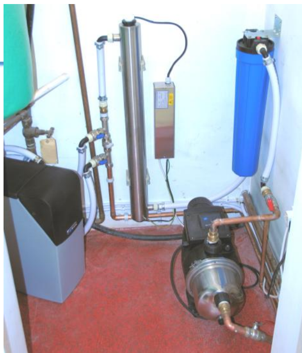
The completed installation. The pump is bolted to the floor. The filter is above it. The UV steriliser and electrics are mounted on the rear wall. The softener is shown on the left.
