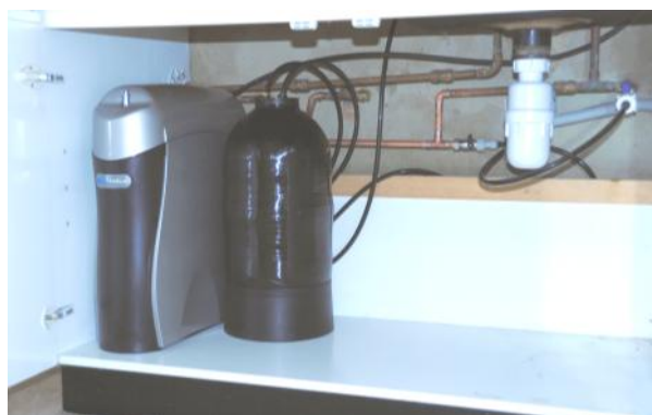
It was convenient to install the reverse osmosis drinking water system under the kitchen sink. New pipe work to the rear feeds bore hole water directly to an outside tap.
