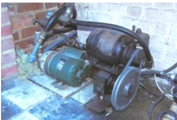
The original pump set up in the property
