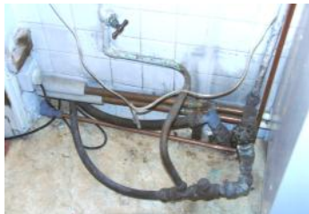
The state of the original plumbing above the bore hole connection
