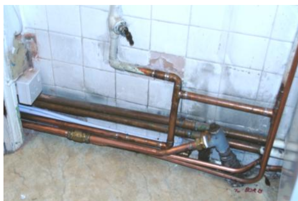
The plumbing above the bore hole (centre right) can be compared with the original set up in the photograph overleaf. The pipe work goes through the wall (left) into the larder cupboard.
