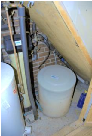
The original softener installed in a cupboard under a staircase
