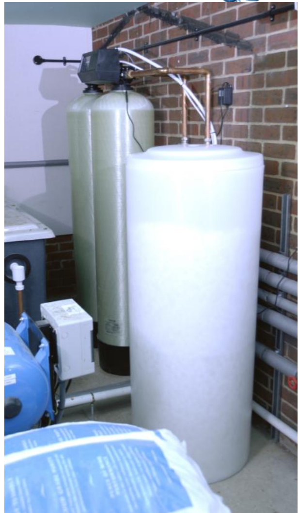
The new 100 litre metered duplex softener, in its final position, in the boiler room with the slim-line salt tank in the foreground.
