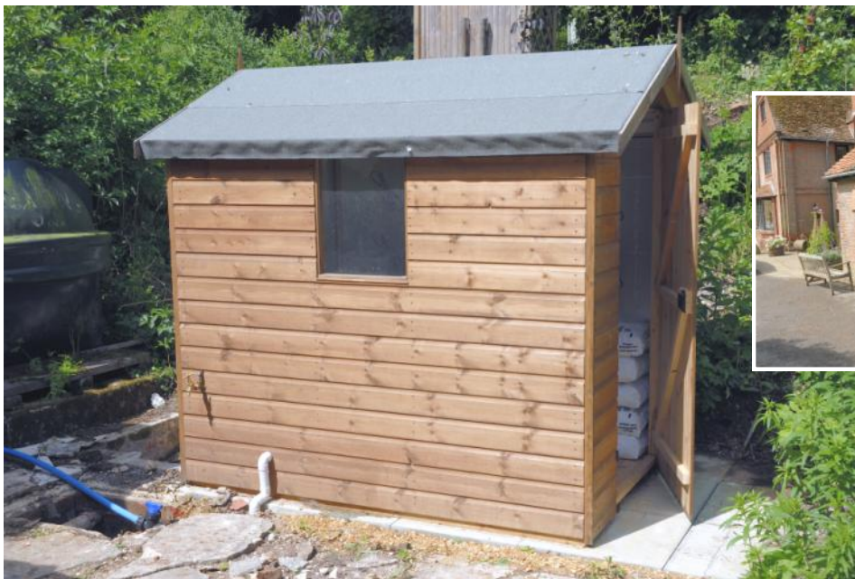
The smaller picture shows where the bore hole is located next to the Jacobean farmhouse. The main picture shows the shed located to rear of the property in which the water treatment equipment is located.
