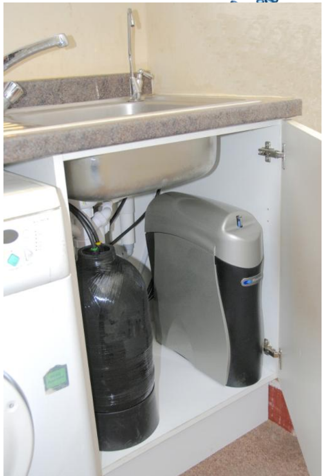
The reverse osmosis system was located under the kitchenette sink along with the storage tank for the pure water. The separate drinking tap is located above. A pure water feed is connected to the medical room on the first floor (see photograph overleaf).
